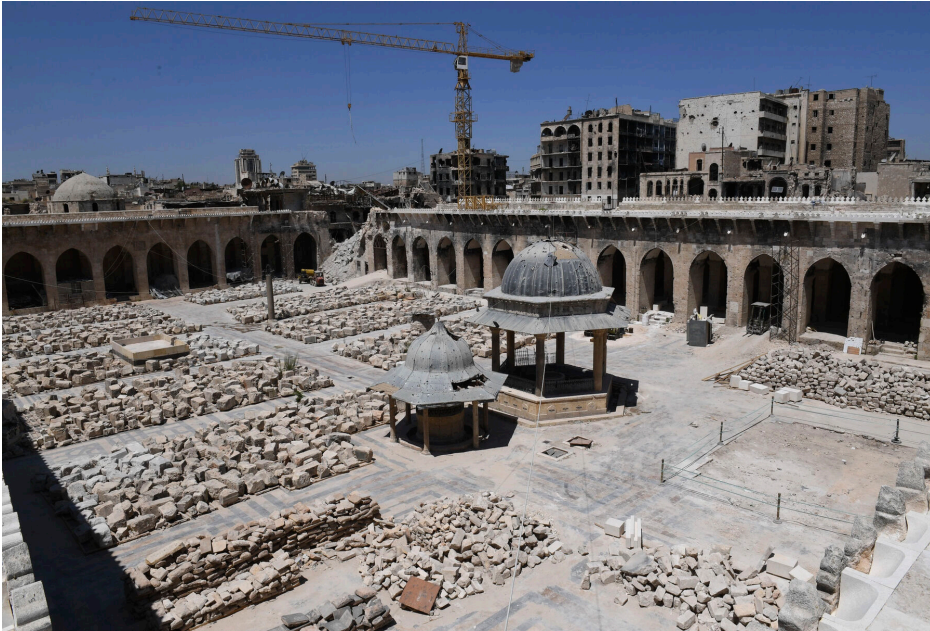
Figure 12.2 Restoration work underway at the Great Umayyad Mosque in the Old City of Aleppo, 14 August 2018. A crane stands over the rubble of the toppled thirteenth-century minaret, whose stones have been catalogued and organized in the mosque's courtyard. Image: George Ourfalian/AFP/Getty Images
